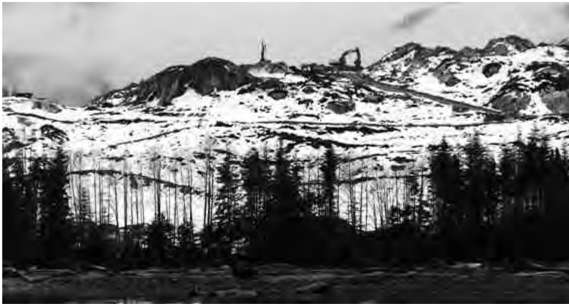
Projects like the Kitimat LNG Project (construction site pictured) could send gas west instead of east through the mainline
